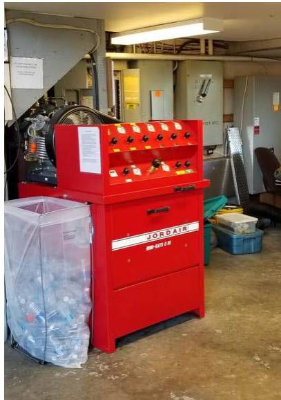
Figure 4: Firefighters are forced to share spaces with various other operations, some of which represent a health hazard. In this case, the high-pressure air compressor is located in an open floor area in the work areas used by firefighters.
